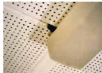
Asbestos insulating board ceiling tiles
