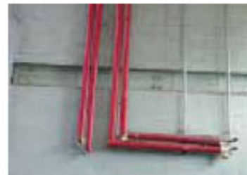
Asbestos lagging on pipes
