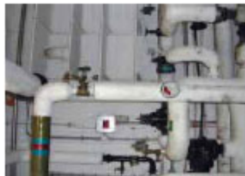
Asbestos insulation on pipes
