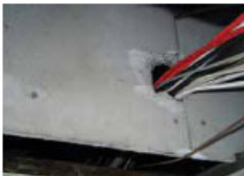
Asbestos insulating board panels
